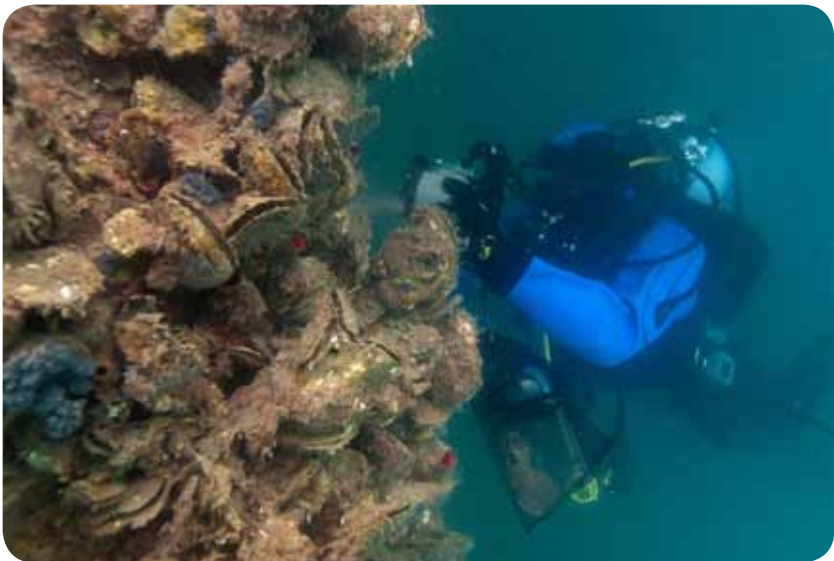
Figure 39: Columns of Koper harbour pier, completely overgrown with epifauna.
