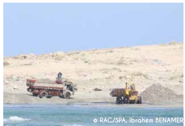
Figure 13. Sand dredging operations with heavy machinery. A truck shown in the picture is loading up sand to be carried to nearby urban areas
