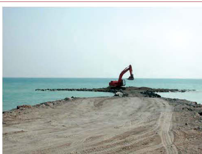
Fig. 65. Borghetto Santo Spirito (Savona province) Building a coastal defence facility (Settore Ecosistema Costiero archives – Liguria region).
