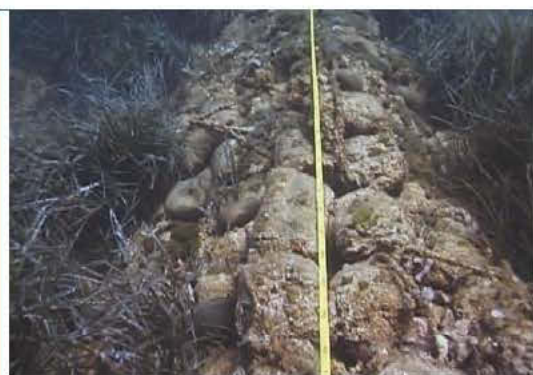
Fig. 114. The electric cable between Corsica and Sardinia, near Cala di Sciumara (Corsica) was laid in 1967. It was fixed over the superficial meadows (10-15 metres) by covering it with little slabs of rock. 35 years later, the impact of this covering has not evolved. The line crossing it is a measuring tape unrolled over the bed during observations. From Pergent et al. (2002b).
