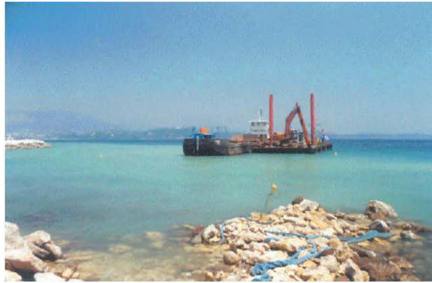
Fig. 72. . A barge and rock-clearing equipment during the digging of an access channel to a port in the Var (France). The turbidity of the water caused by the work is obvious. Photo by P. Bonhomme.
