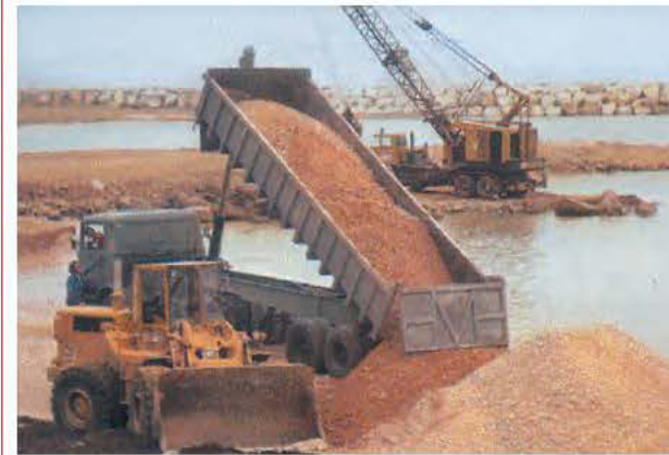
Fig. 58. Developing Le Mourillon's artificial beaches (Toulon, Var, France). A lorry discharging earth directly into the sea.
