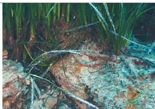
Fig. 115. The electric cable between Corsica and Sardinia, near Cala di Sciumara (Corsica) was laid in 1967. Its hold on the meadows has been reduced by a start of recolonization of the slabs of rock by Posidonia oceanica . From Pergent et al. (2002b).
